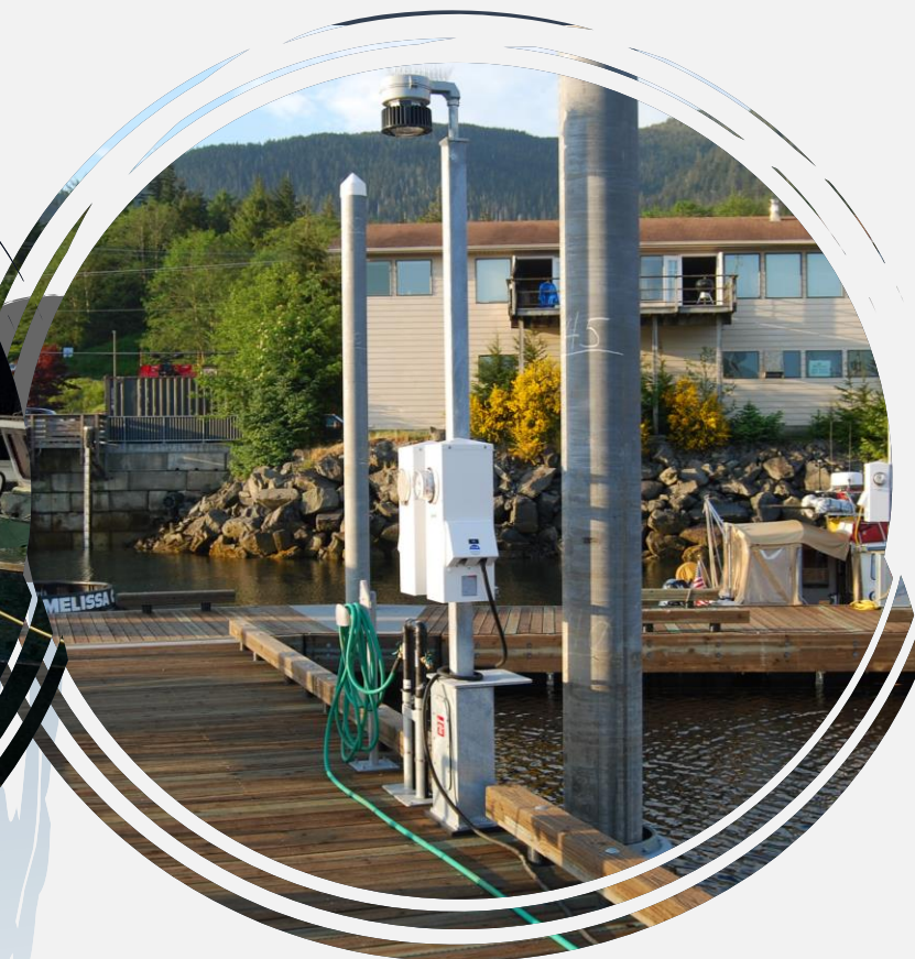
Combined Lighting & Electrical Pedestal
