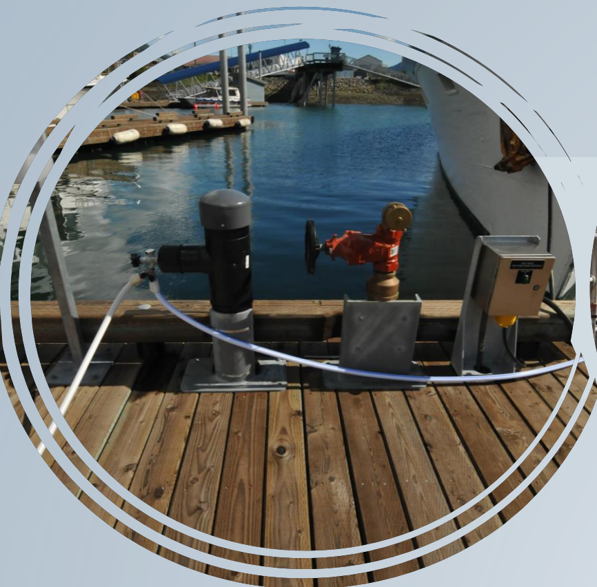
Freeze Protected Water & Fire Suppression Pedestal
